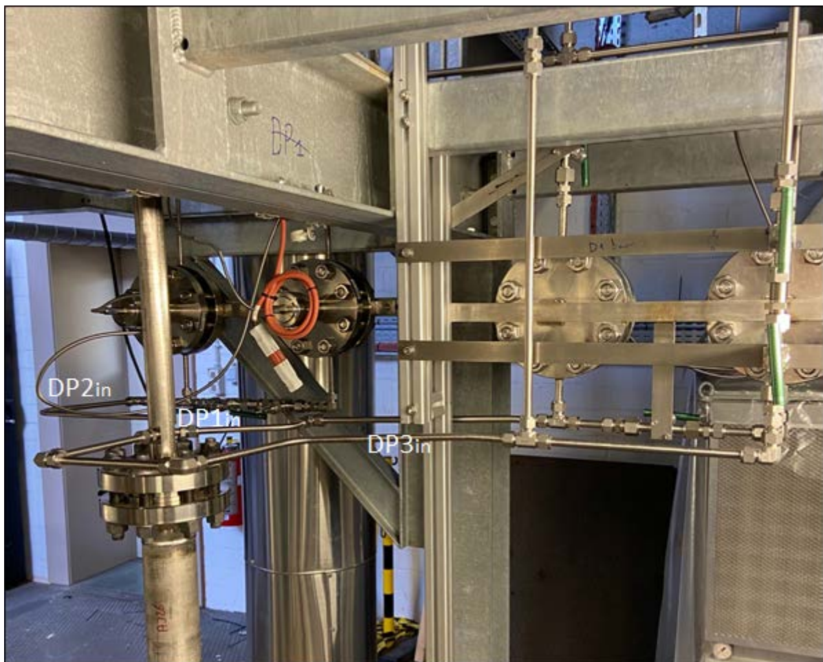
Fig. 17. Inlet tubing pressure station.
