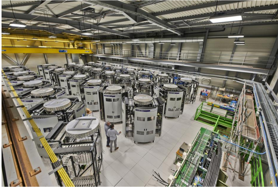
Figure 12: The 2 x 16 towers of the new SPS RF powering installation.
